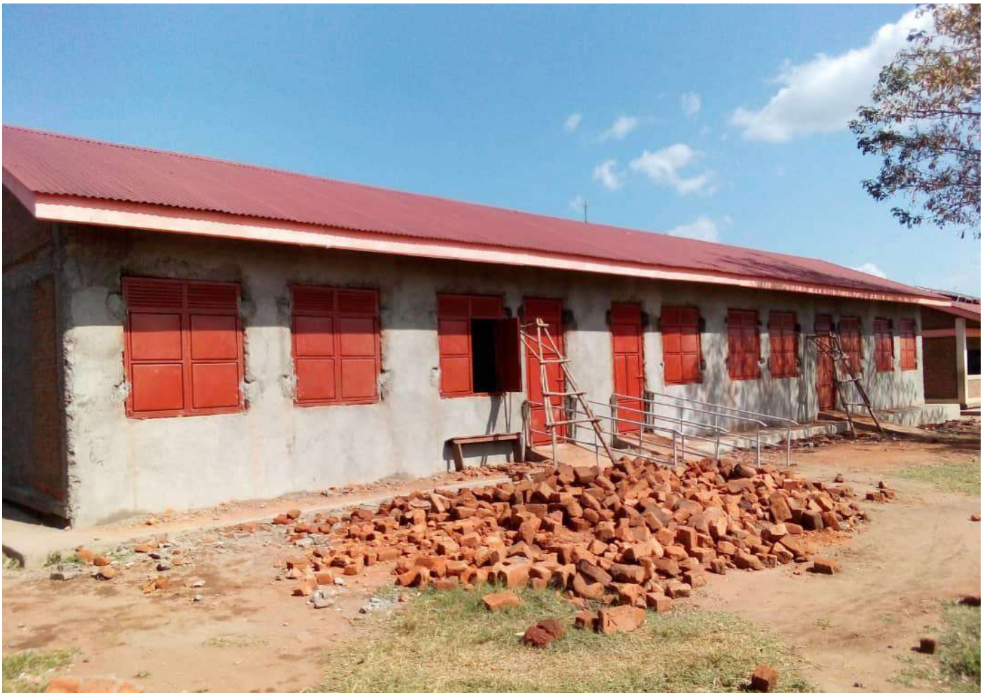
Longamare Primary School in Imvepi Refugee Settlement, Terego district under renovation with support from EQUATE education project.
